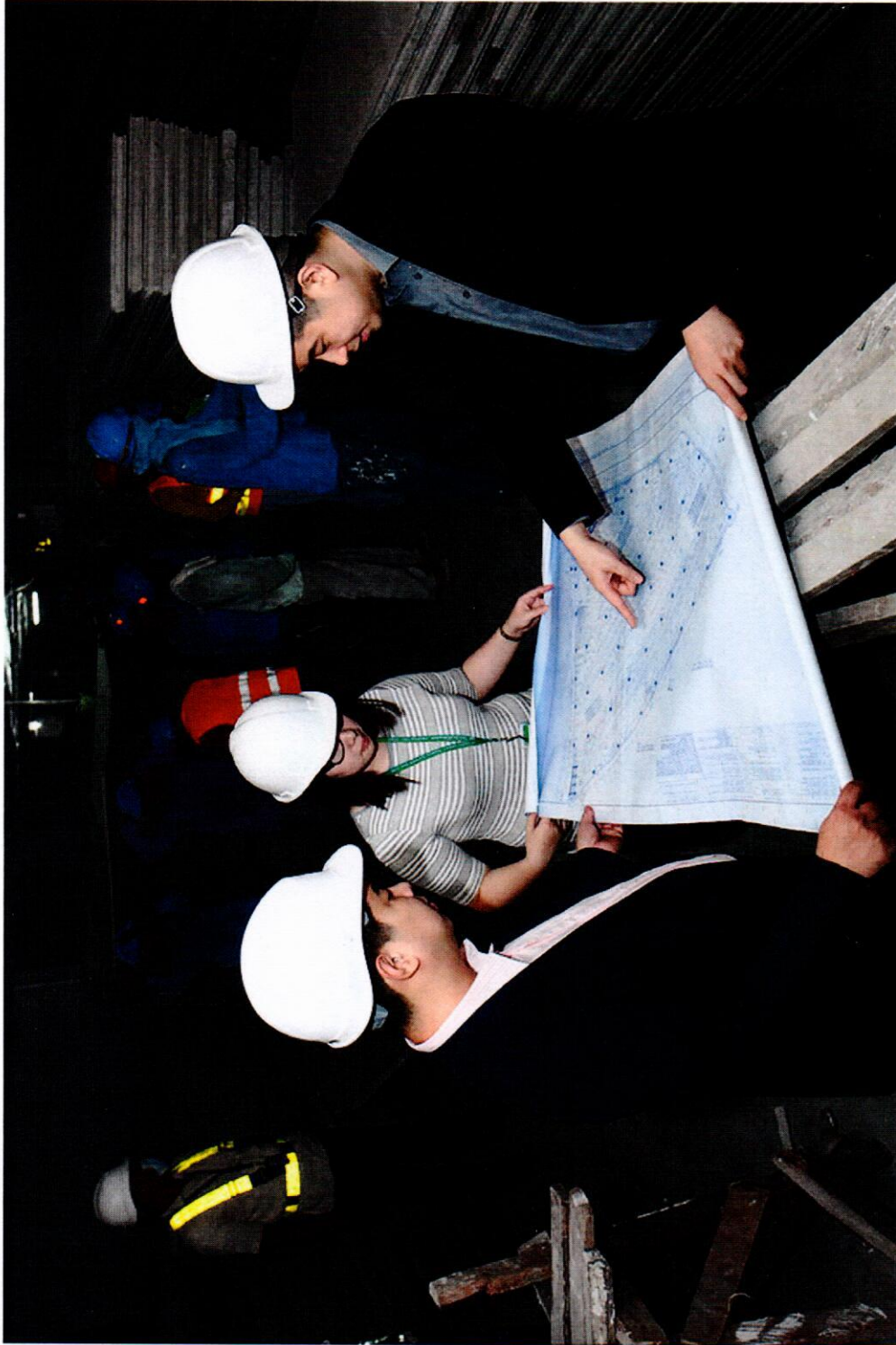
DD Chairman Edgar 'Injap' Sia II together with DD President Ferdinand Sia and DD EVP/CFO Rizza Marie Sia inside the construction site of the soon-to-open Dragon8 Shopping Center in Divisoria, Manila
